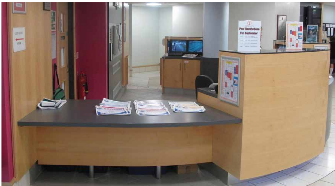
Reception counter with lowered and standing height sections (Amphitheatre Wellness Centre, Carrickfergus)
