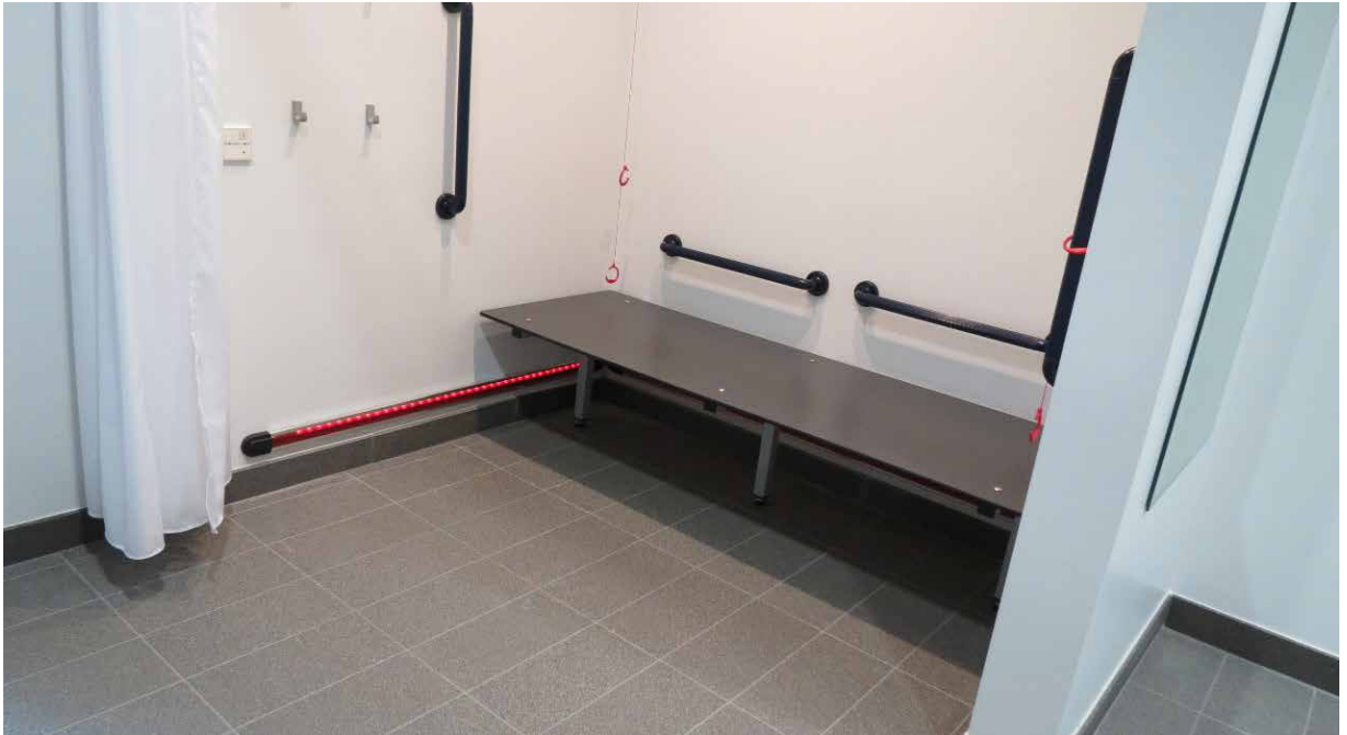
Wheelchair accessible incorporated changing provision within inclusive changing area (Foyle Arena, Derry-Londonderry)
