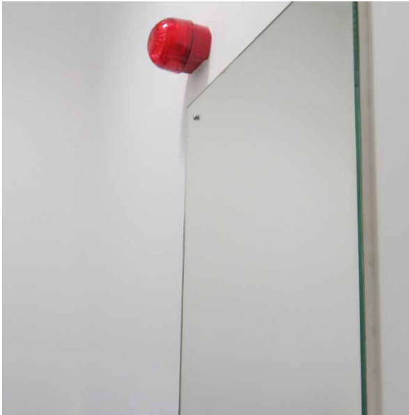
Use of flashing beacon alert within self-contained unisex wheelchair accessible WC unit
