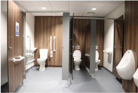
Image 3 - Wheelchair accessible WC cubicle and ambulant accessible WC cubicle incorporated within an inclusive toilet block
